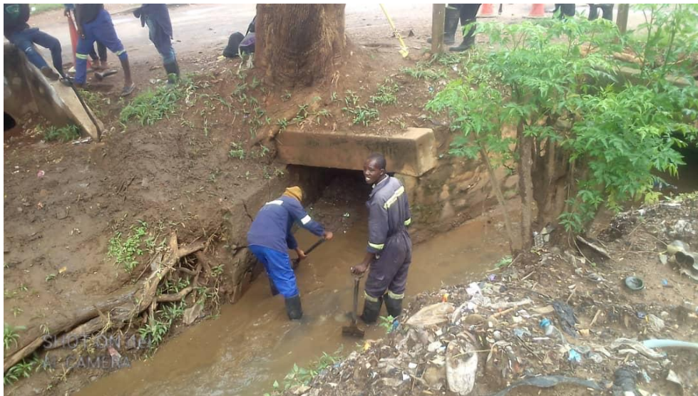
Figure 6: Shows the unblocking of drainage system in the CBD- Kabwe. (pictures from engineering Department Kabwe Municipal Council)
