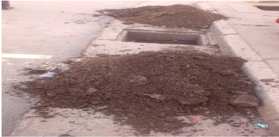
Figure 8: Shows Silt and debris removal from underground drainages. Kabwe (CBD) (pictures from engineering Department Kabwe Municipal Council)
