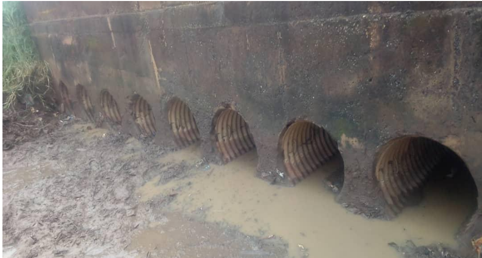
Figure 7: Shows unblocked drainages which were silted due to Capacity. Kabwe (CBD). (pictures from engineering Department Kabwe Municipal Council)
