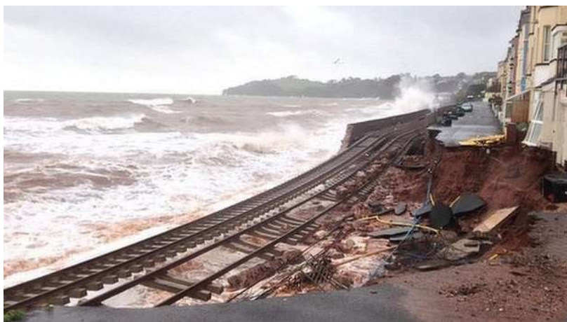
Damaged railway line at Dawlish. Photo courtesy BBC
