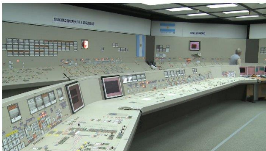
Photo: Main Control Room of the Nuclear Power Plant “Atucha II”.
