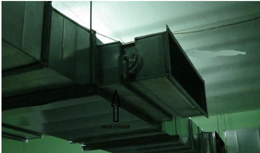
Figure.2. Air Duct for Exhaust system
