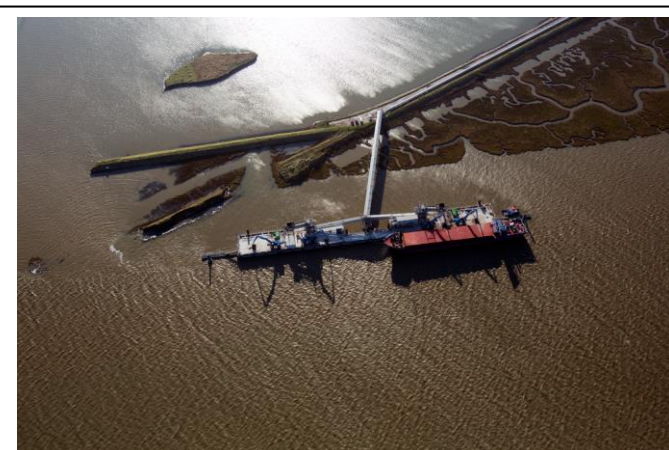
Purpose built jetty for transfer of spoil from southern Crossrail tunnels. Photo: Crossrail
