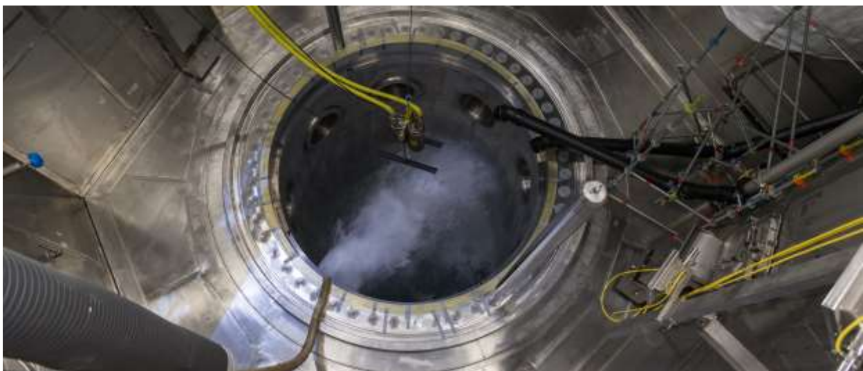
In the photograph: Flushing of the Olkiluoto 3 primary circuit (photo courtesy TVO)
