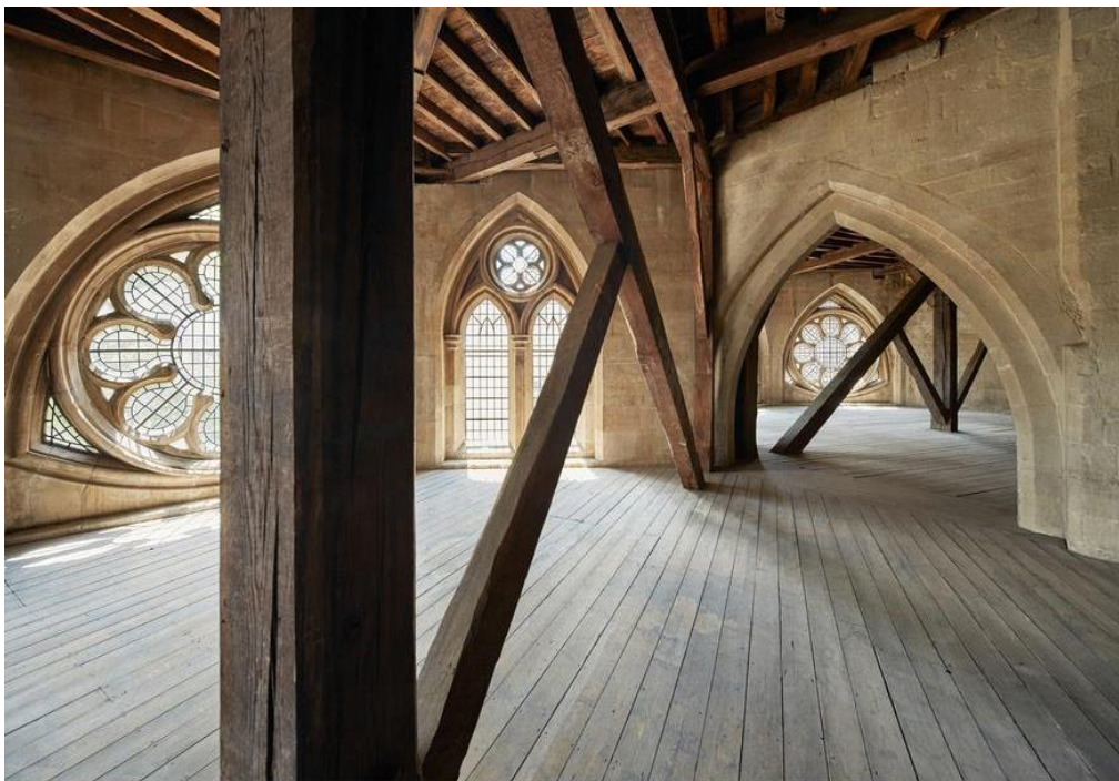
The triforium at Westminster Abbey before work began to convert this space, hidden from the public for 700 years, into a new museum: The Queen's Diamond Jubilee Galleries. Picture: Alan Williams
