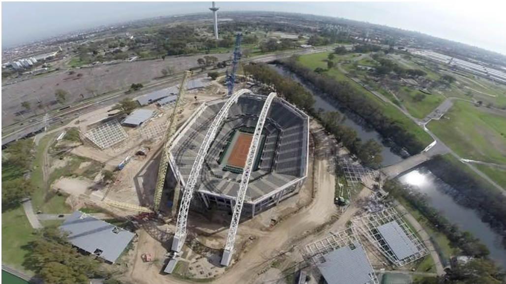
Photo: Roofing Project of the Mary Terán de Weiss Stadium, one of the venues of the Olympic Games.
