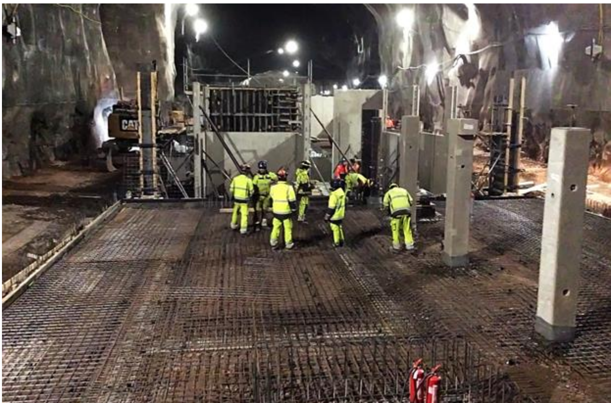
Soukka station prior to casting of the station platform floor (photo courtesy Länsimetro)
