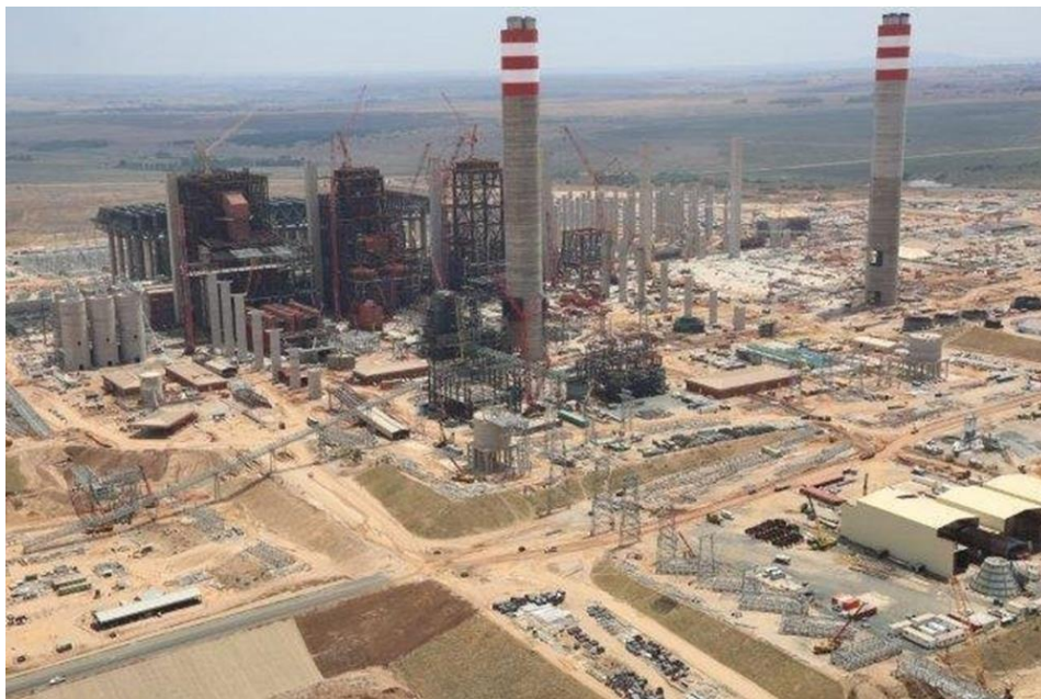
Figure 1 – Kusile Power Station Aerial Photograph (Dec 2016)
