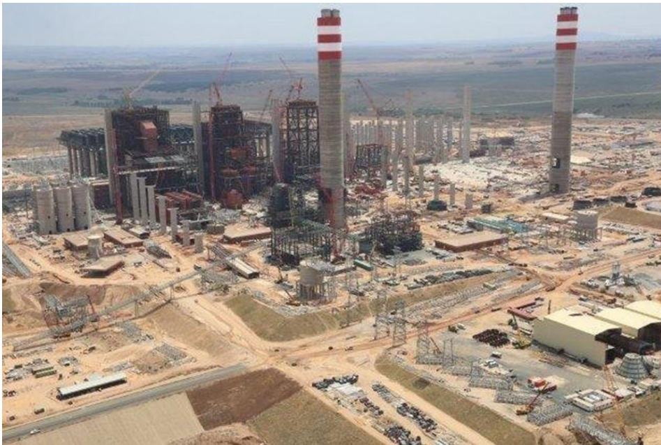
Figure 1 – Kusile Power Station Aerial Photograph (Dec 2016)
