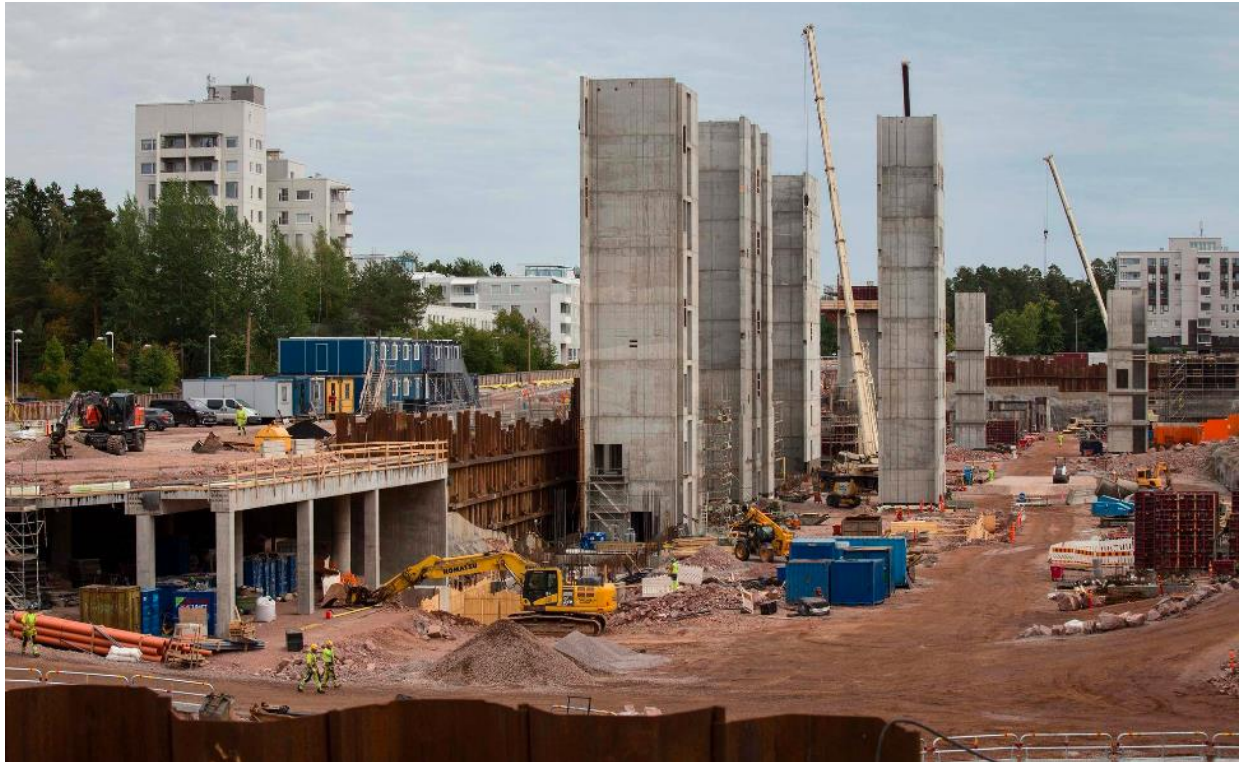
Construction of Lippulaiva shopping center at the Espoonlahti station (photo courtesy Kaveh Rostamkhani / HS)
