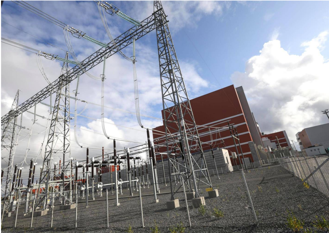
Olkiluoto 3 plant at Eurajoki, Finland (photo courtesy Seppo Kärki)
