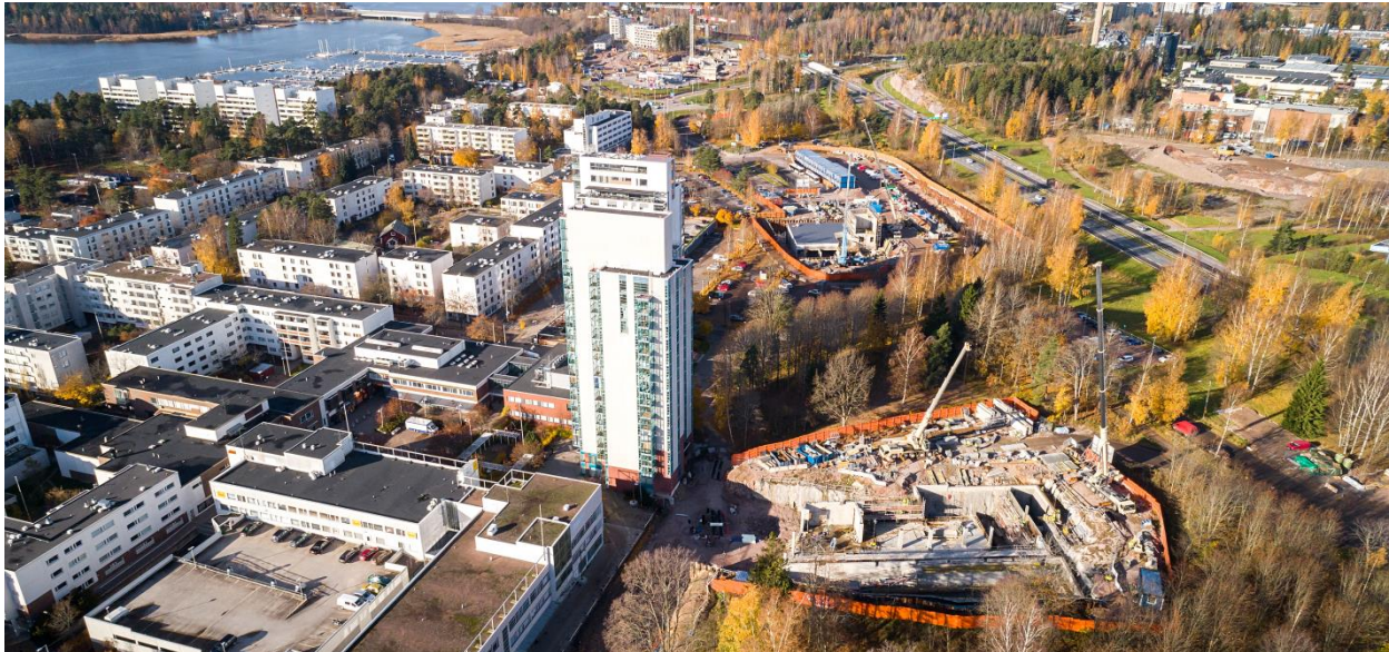
The construction sites at the Kivenlahti station (photo courtesy Iiro Mikola / Optivision)
