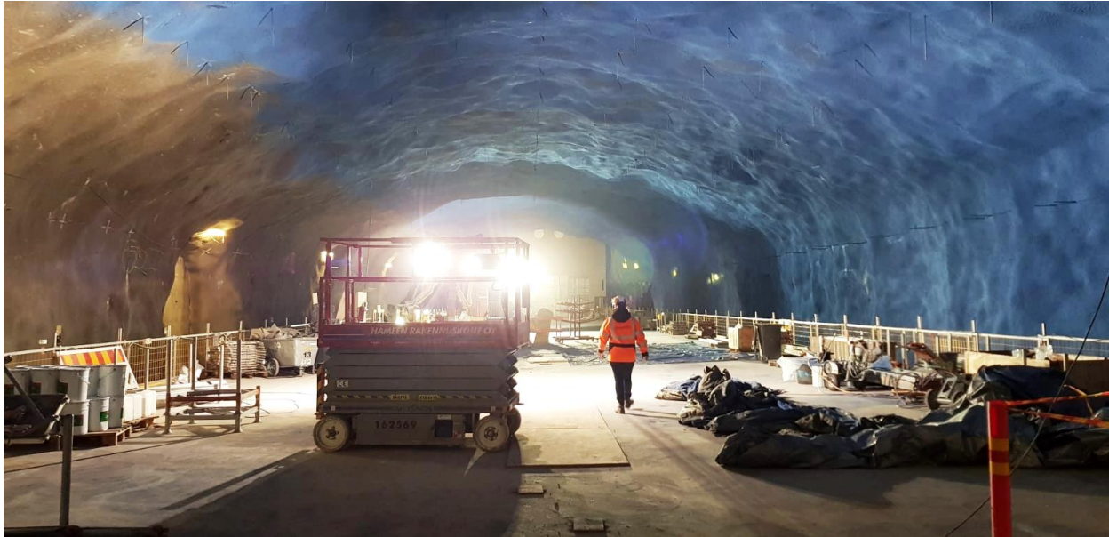
Espoonlahti station hall with ceiling painted blue (photo courtesy T. Virtanen / Länsimetro)
