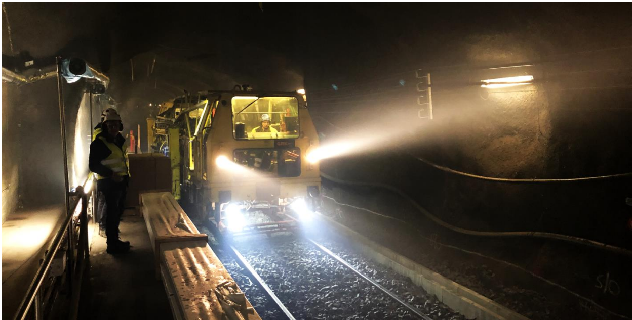
Tracks are being laid at Länsimetro second extension (photo courtesy S. Natunen / Länsimetro)
