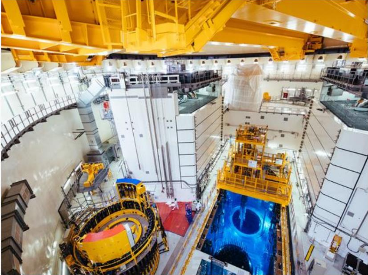
Nuclear fuel loading about to commence in Olkiluoto 3 reactor building (photo courtesy TVO)
