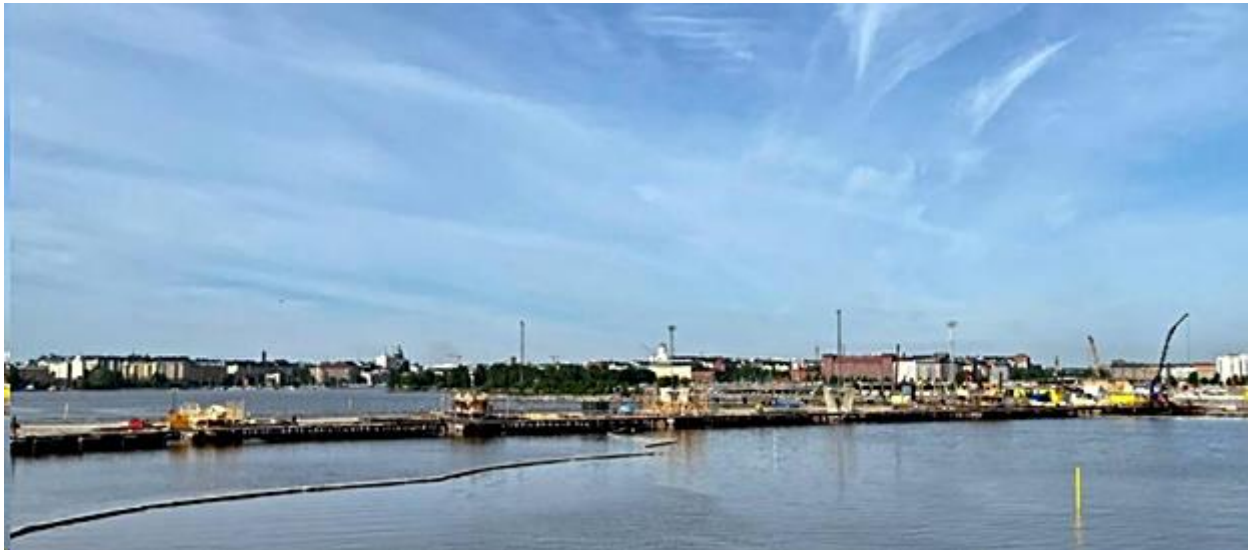
A temporary construction bridge, with downtown Helsinki in background (photo courtesy Sanna Hellström)
