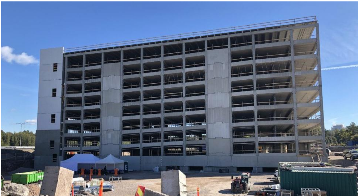
New car park facility next to the Kivenlahti metro station (photo courtesy M. Partanen)
