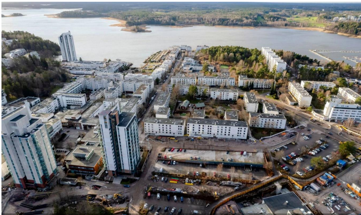
Aerial view of Kivenlahti, with the metro station construction site at the bottom (photo courtesy Kalle Koponen / HS)
