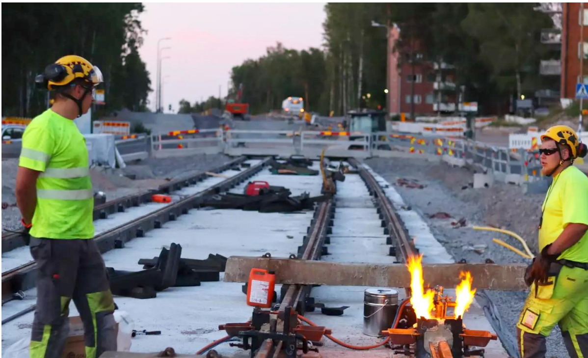
Welding tracks in the dead of night to avoid thermal expansion (photo courtesy Raide-Jokeri)
