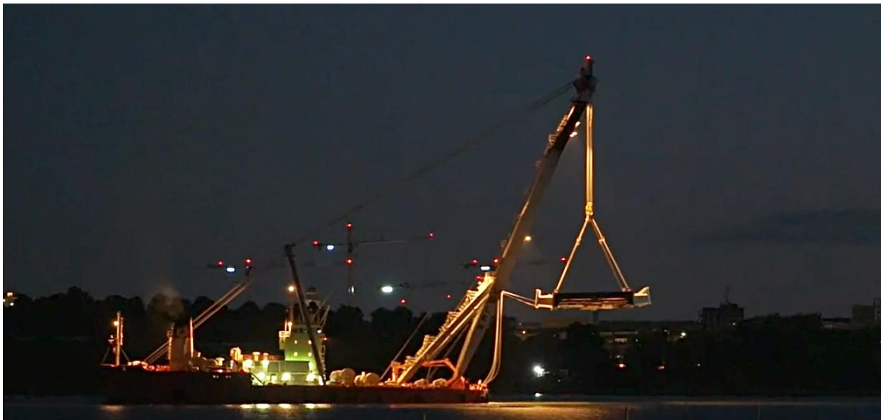
HLV Uglen lifting one of the main steel sections at night (photo courtesy vesselfinder.com)
