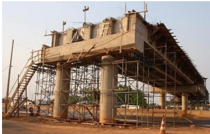
Photo: Stalled construction
