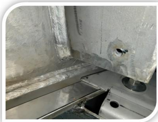
Figure 10: Support Rings Misalignment
